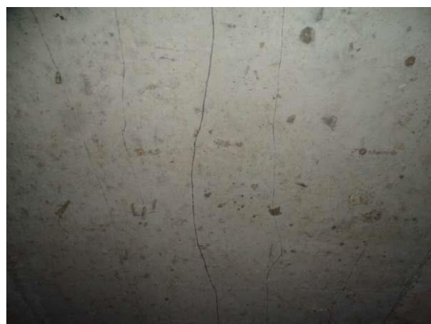
(a) 左幅箱内顶板纵向裂缝
