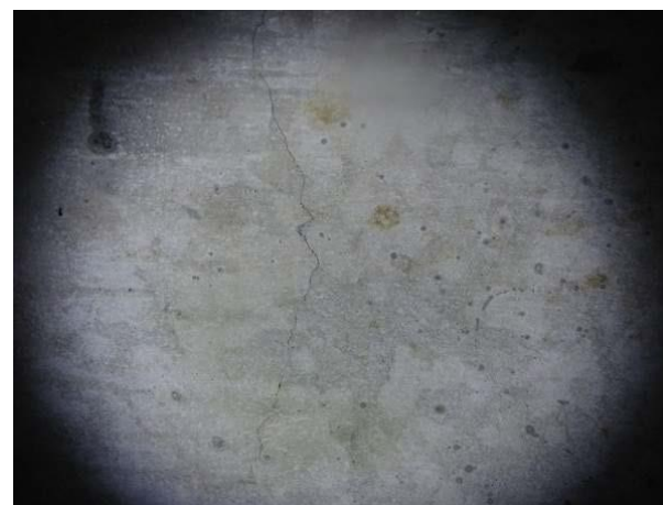
(a) 左幅箱内顶板纵向裂缝
