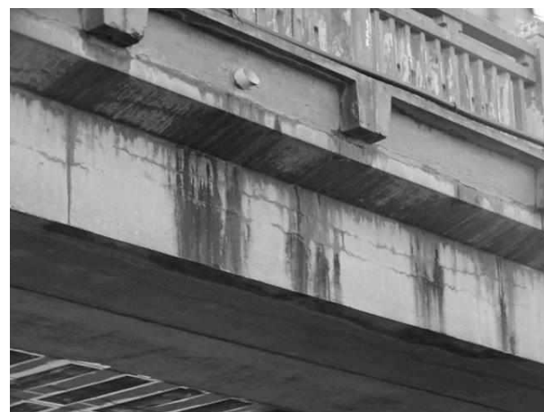
(a) 4-9#空心板右腹板纵向裂缝
